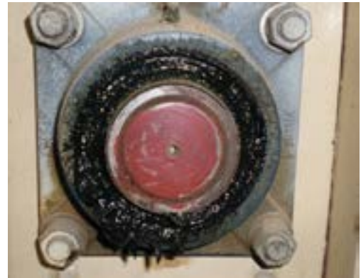
Overgreasing can result in higher operating temperatures, premature bearing failure and an increased risk of contaminant ingress.
