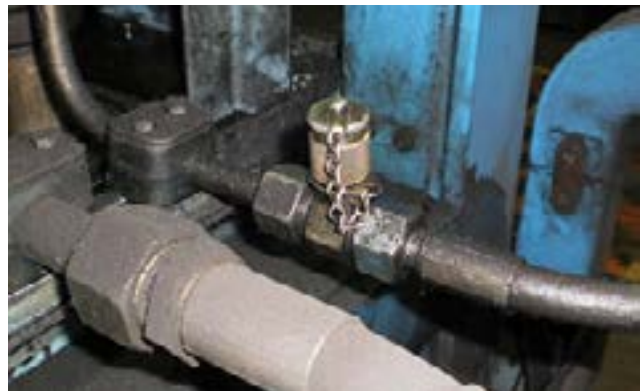
Improper sampling points and hardware may result in samples that are full of historic data.
